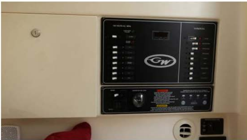
The main switch panel is located at the aft bulkhead of the starboard console.
